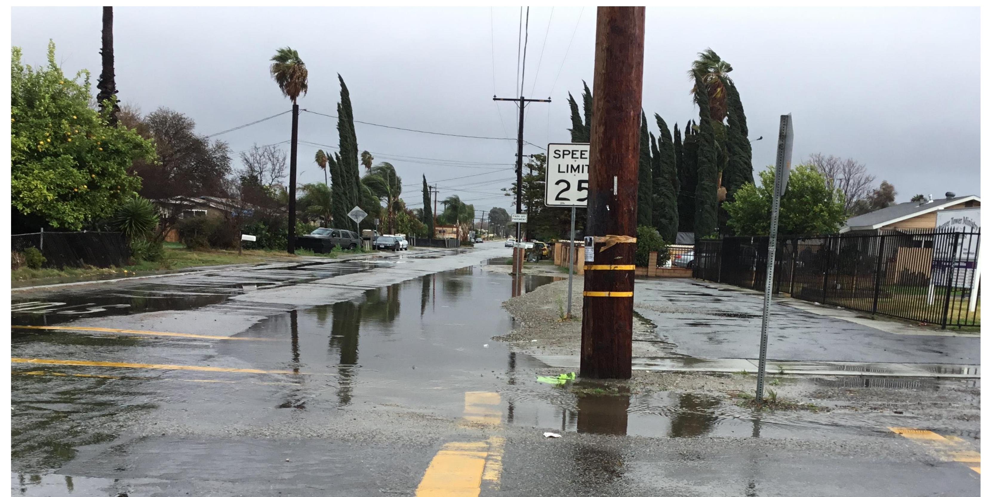
Figure 1: 9 th Street and Kadota Ave Intersection after a large rainstorm.
