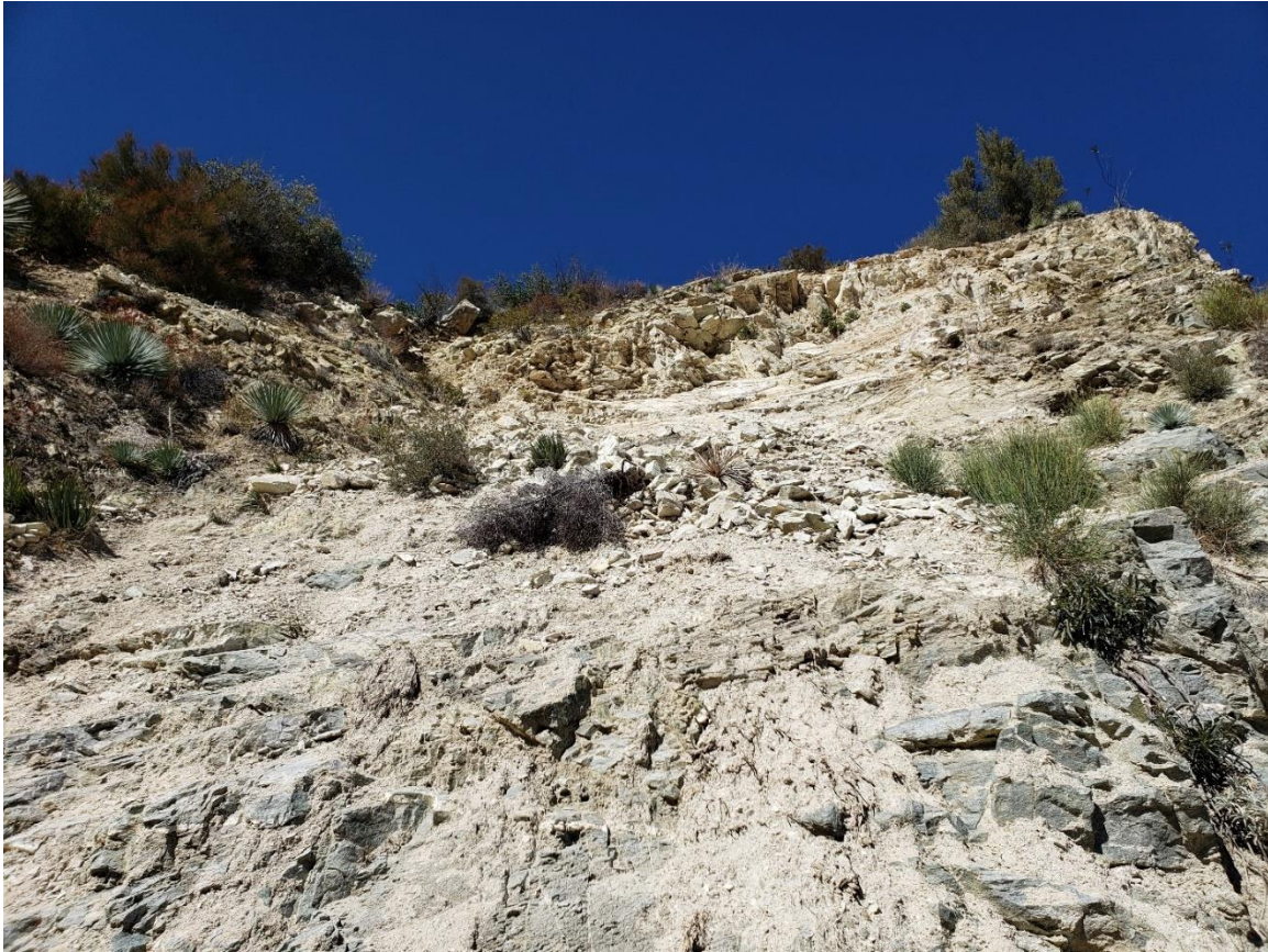
Figure 84: Photograph showing the LS3 failure surface up above.
