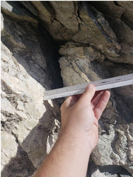
Figure 32: Fracture about 1.5 inches wide under the lookout.
