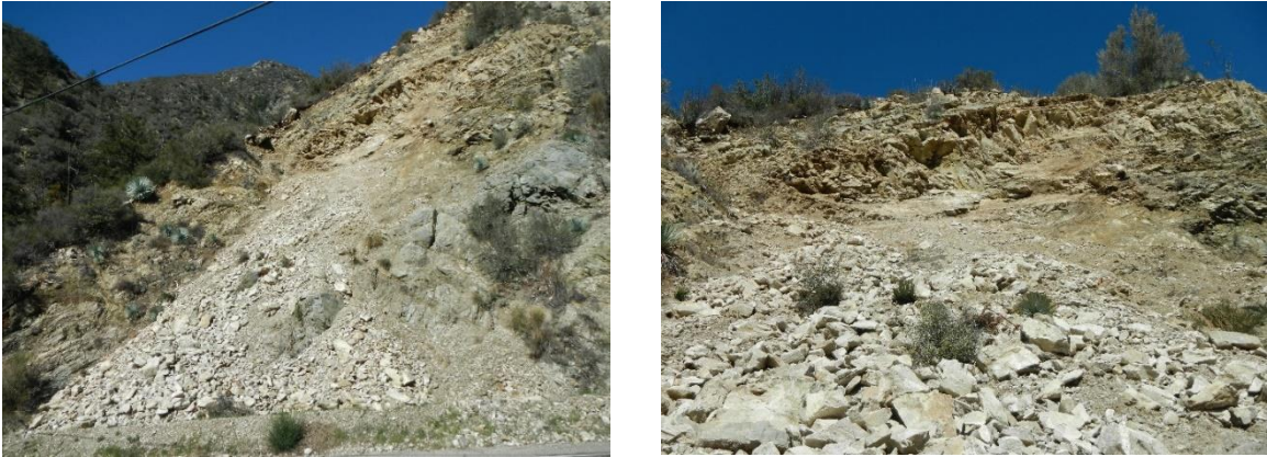
Figures 34 and 35: Photos showing the failed landslide surfaces taken on February 11, 2019, by Dr. Nourse.
