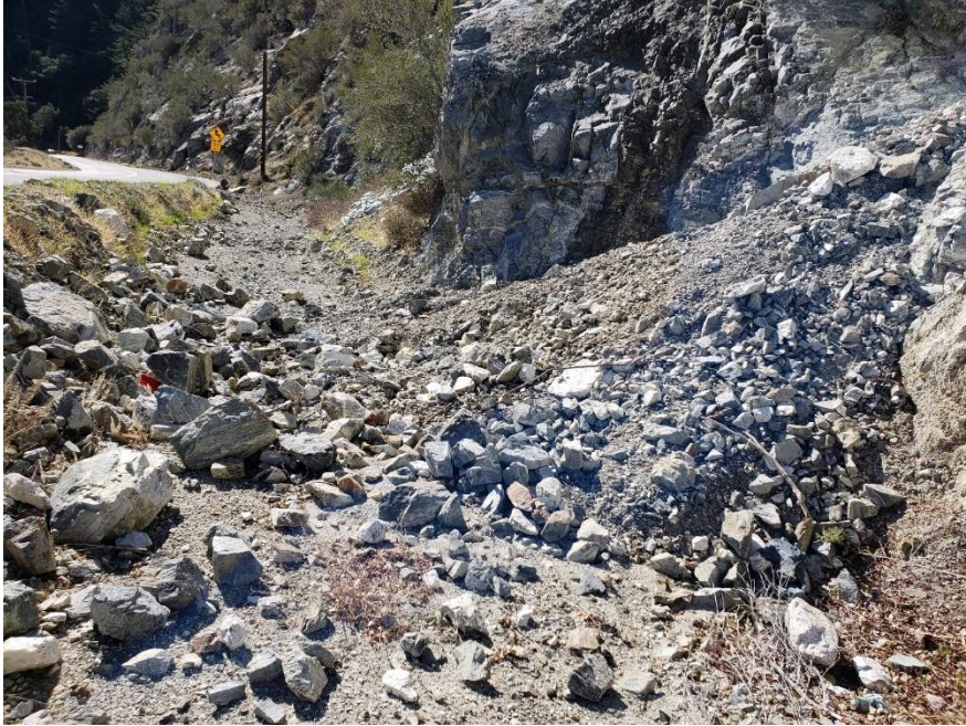
Figure 31: View looking south to the debris cone after winter storms from above wedge LS1 taken on 1/19/19.
