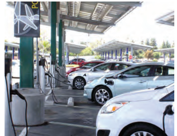
EV charging stations.
