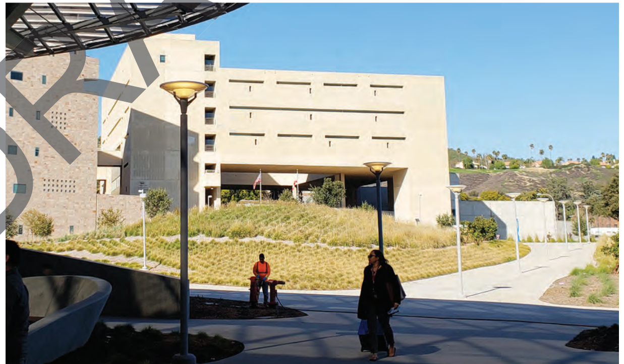
Bldg 98C exterior will be replaced with a new envelope, designed for enhanced energy efficiency and fully enclosing the raised plaza space.
