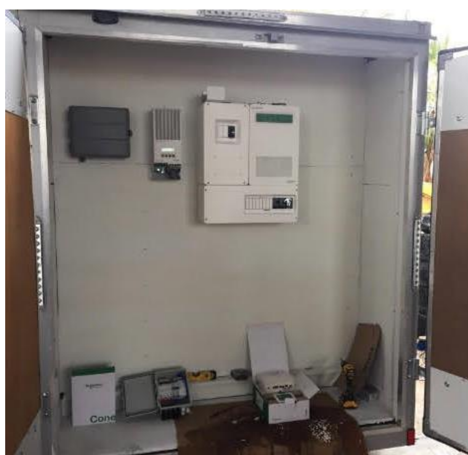
Inside electronic component compartment.
