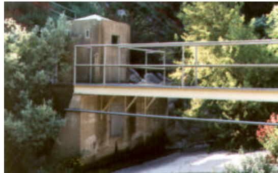
Figure 6 - A photograph of the Big Dalton stream gauge. Electric monitoring equipment is located inside the tower to the right of the photograph. A measuring tape for visual inspection of runoff is secured to the wall below the bridge.
