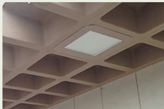
CSU Dominguez Hills LED lighting
