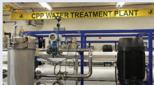
Cal Poly Pomona water treatment plant
