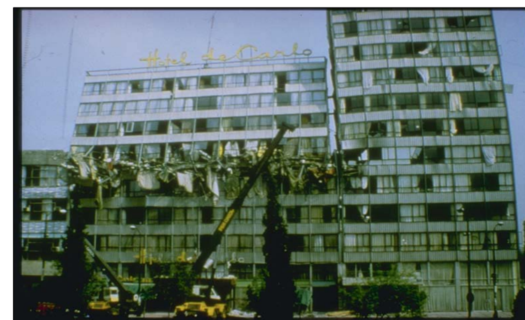
Fig. 1 - A case of structural failure due to pounding in Greece Earthquake of 1978
